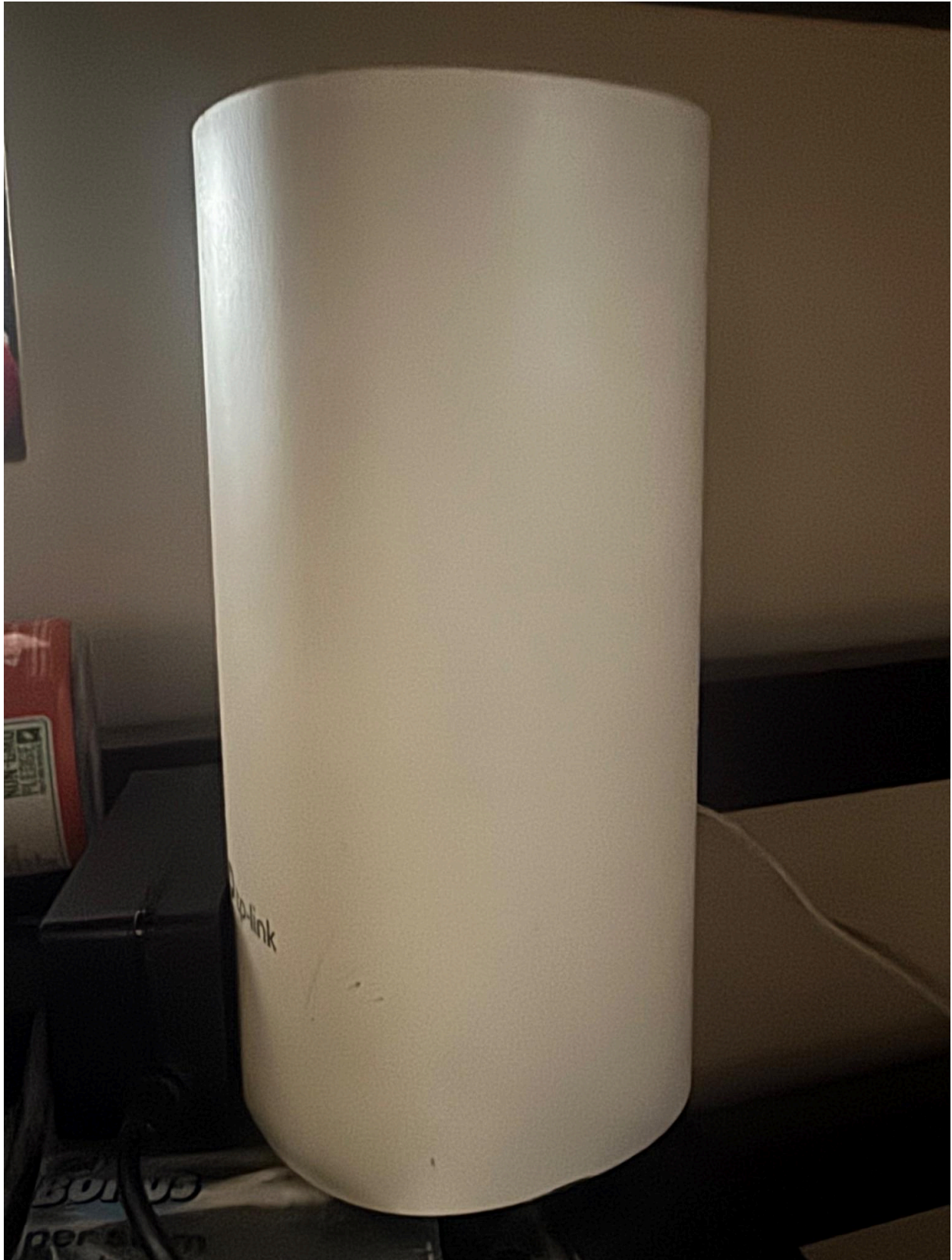
Figure 11. Topology status; TP-Link Primary WiFi Repeater inside main room clean; no issues
